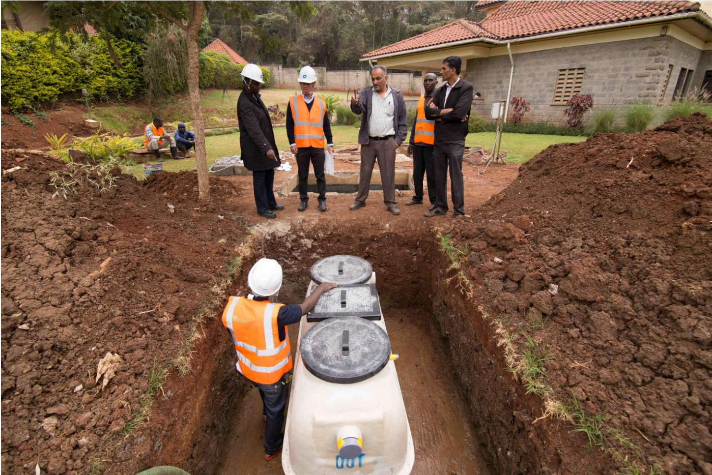
Small scale Johkasou installation_1m3/day
