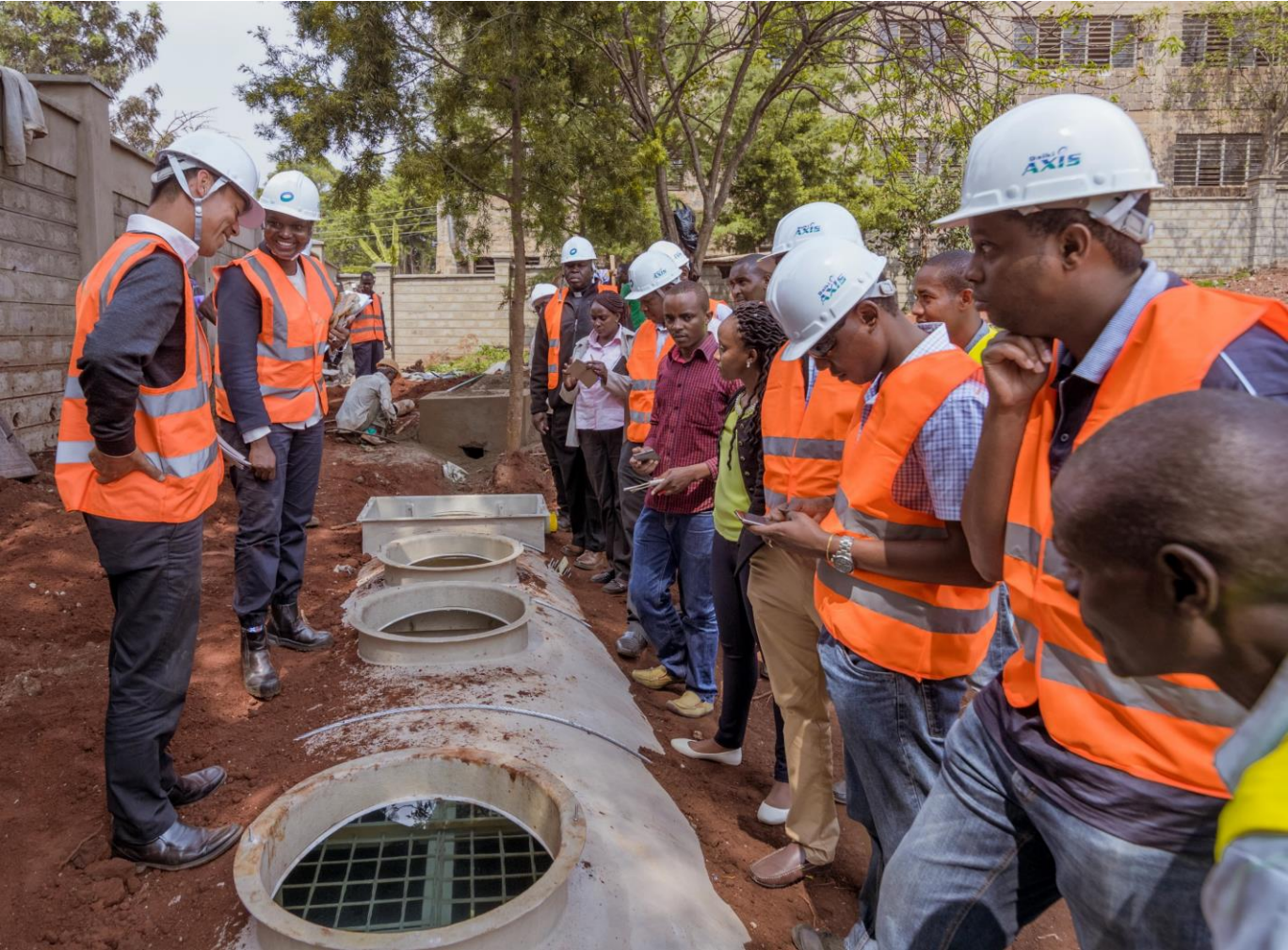
Johkasou introduction at the installation site
